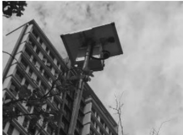
Solar panels used at a project site
